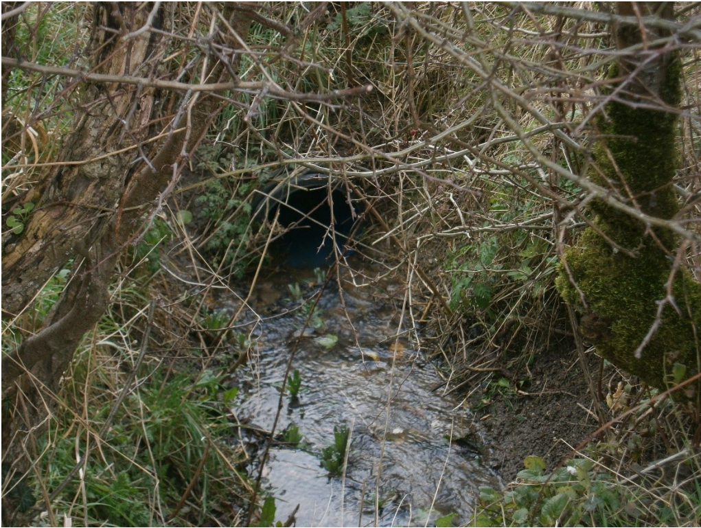
Photograph no. 11. Common Road end of piped ditch opposite “Old Orchard” on 21 February 2022.
