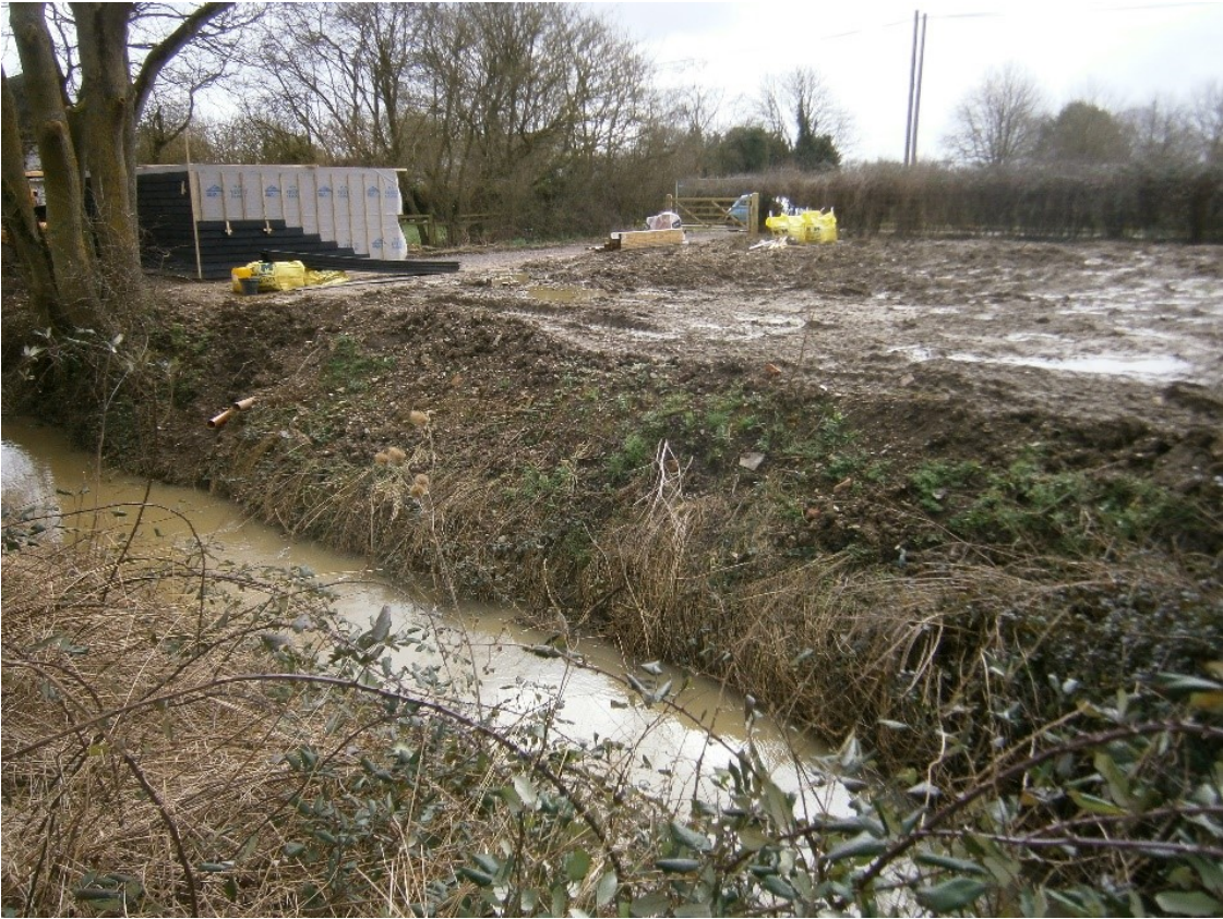
Photograph no. 5 taken of land adjacent College Farm on 21 February 2022. There had been some rain in the preceding days. Note the level of the site compared to the land beyond in photograph no.6 below.
